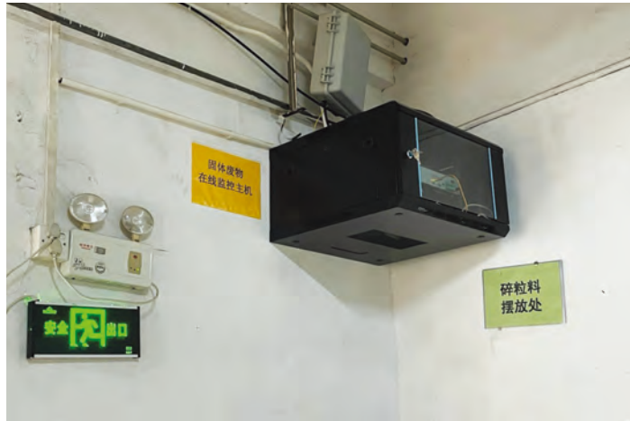
Online Monitoring System for Solid Wastes 固體廢物線上監控系統
